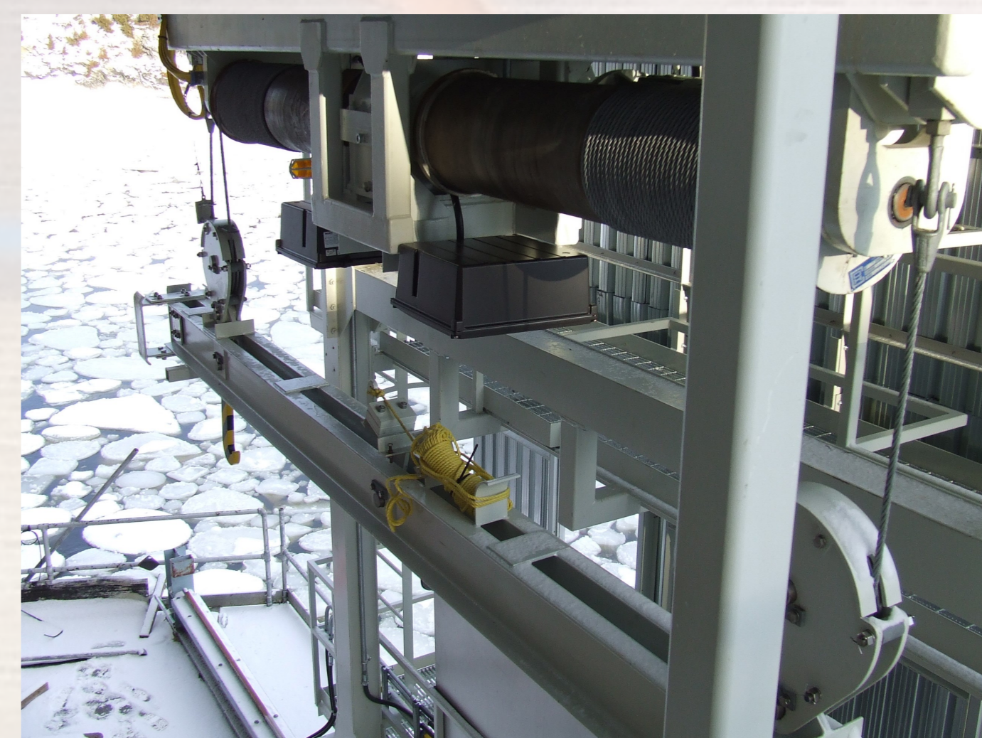
Lifting Hoist and Lifting Beam Downstream Gantry Crane After
