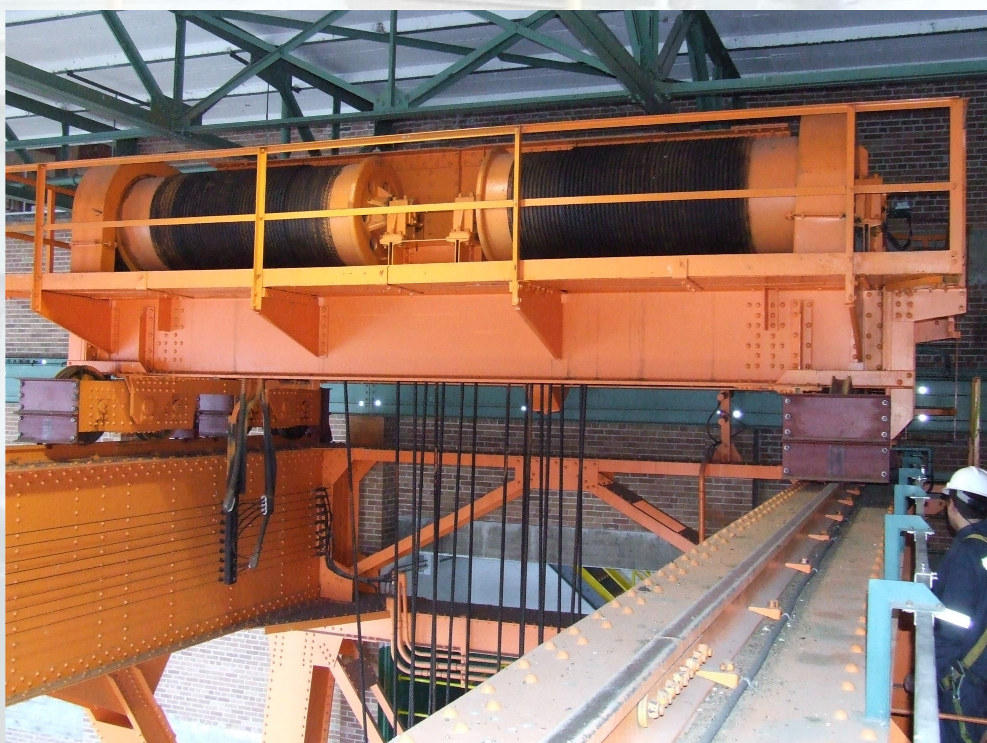
Hoist of the Gantry Crane in the Powerhouse Before
