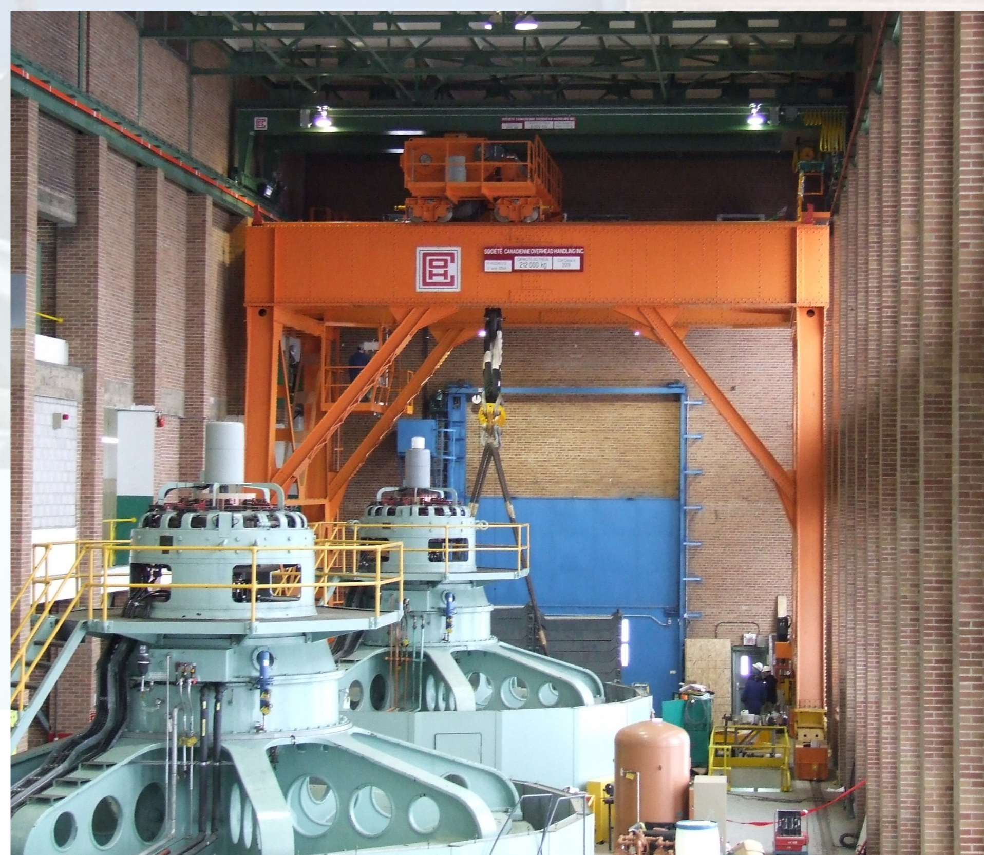
Gantry Crane in the Powerhouse (234 tonnes) After
